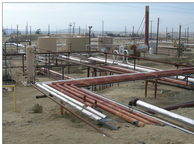
Figure 3: Steam Distribution & Oil/Water Collection At Seneca's Lost Hills, Heavy Oil Production Field
