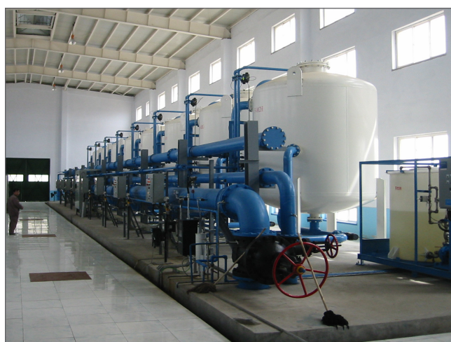
Figure 4: Spectrum Micro Media Filters on Site is a Key Factor in Produced Water Treatment at the Liahoe Heavy Oilfield in China
